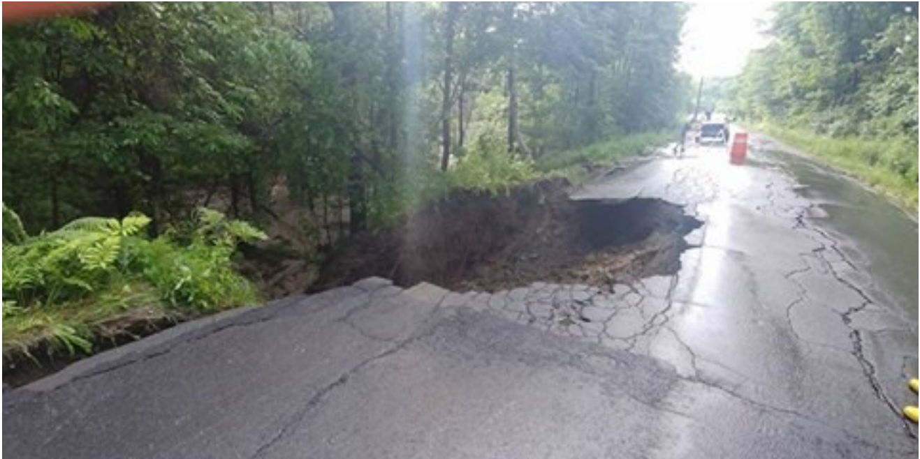
Indian Pond Road Washout Photo Credit: Town of Piermont
