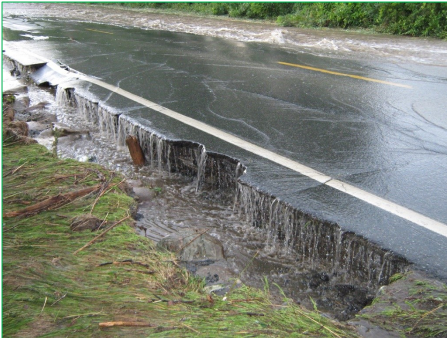
Flooding NH Route 10, July 1, 2017 Photo Credit: Town of Piermont
