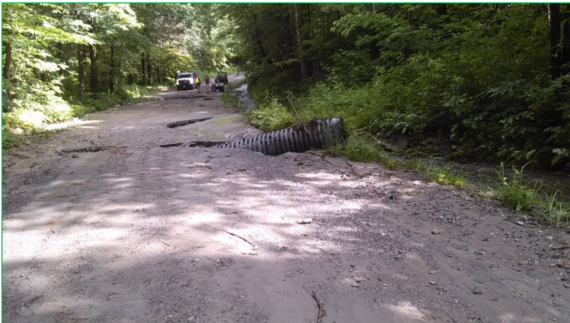
Cape Moonshine Road damage, July 1, 2017 Photo Credit: Town of Piermont
